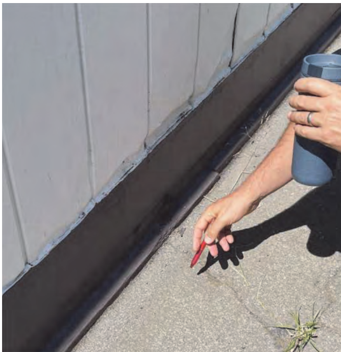
Damage to Plywood Skirting
