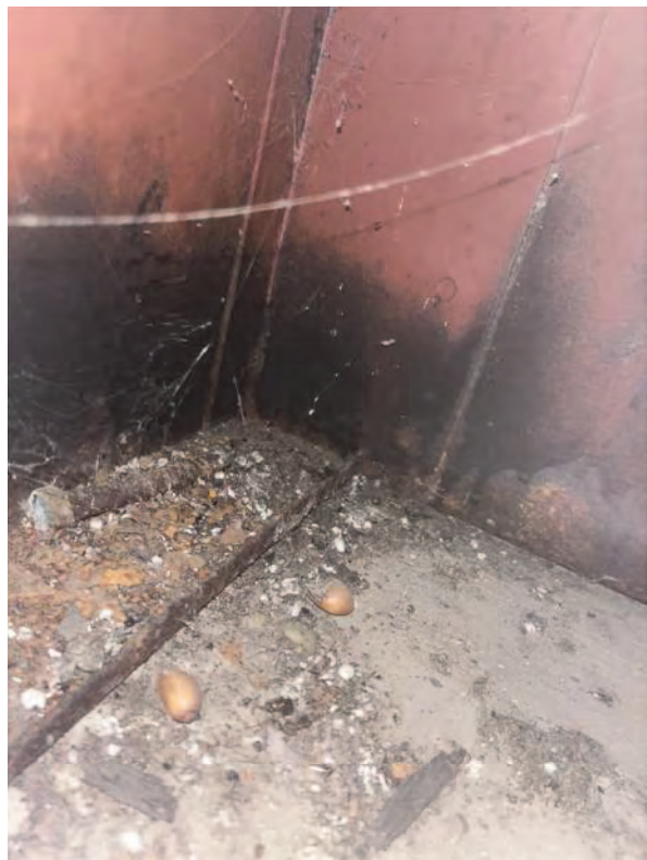
Slight Deterioration of Floor System on Footing
