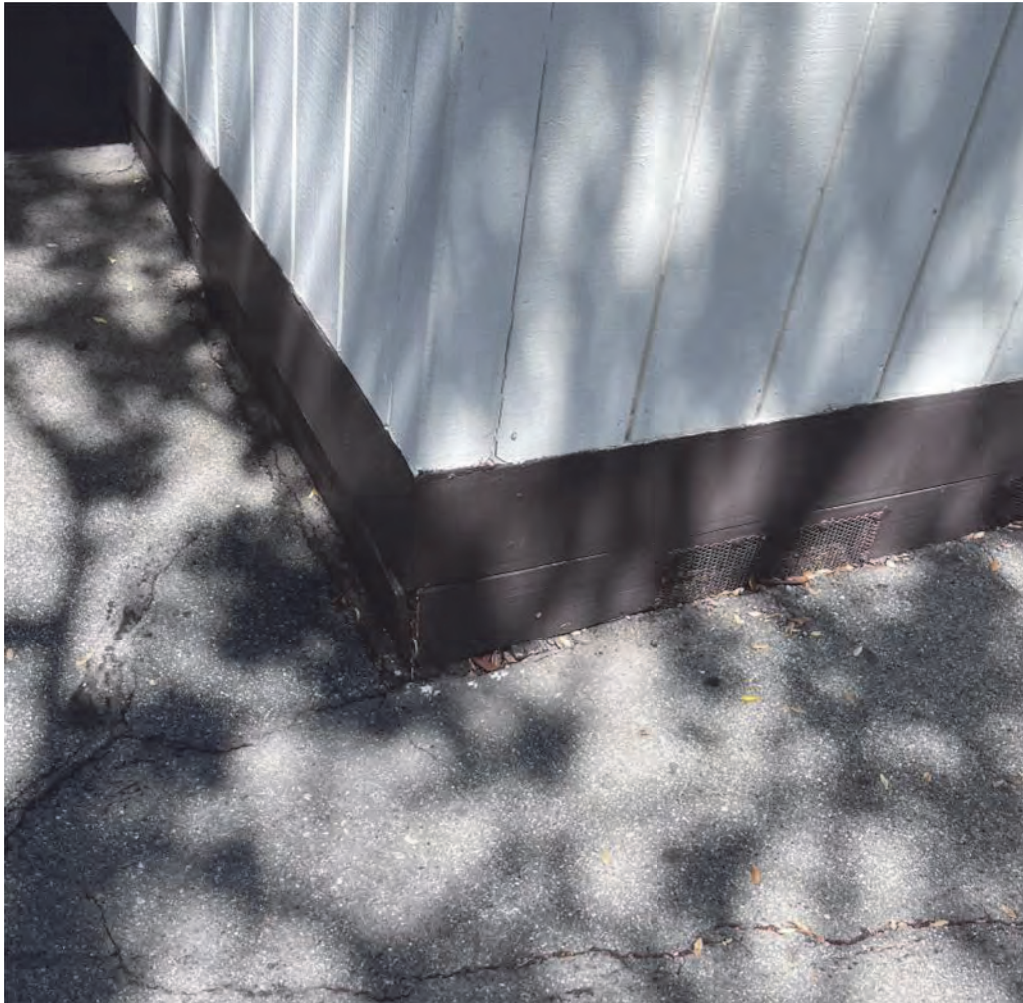
Slight Deterioration of Wood Sill-On-Ground and Cripple Wall Sheathing
