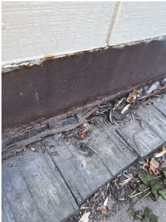
Damage to Plywood Skirting/Wood Sill
