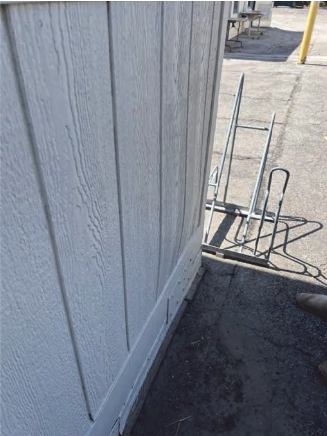
Damage to Metal Framing @ Foundation
