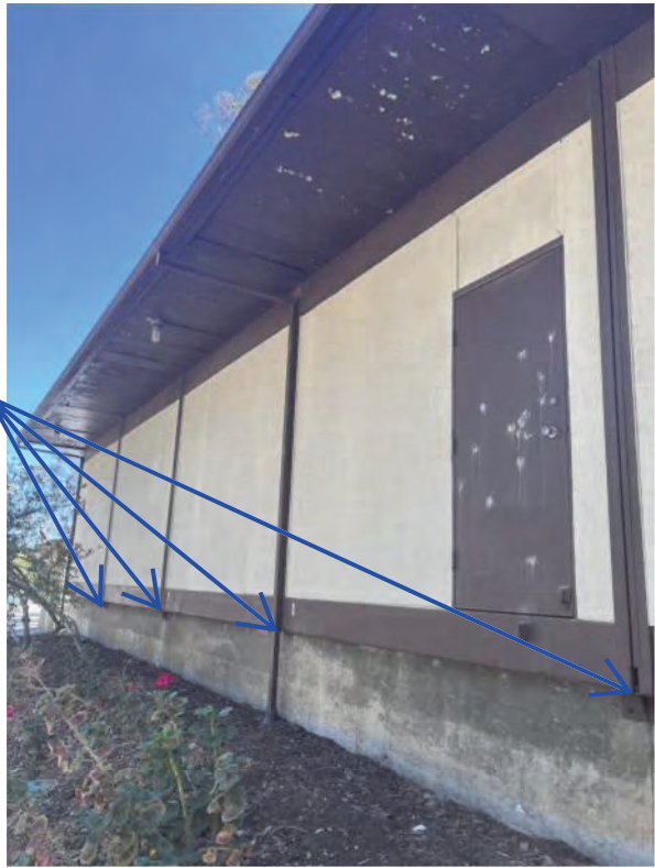
Inadequate Footing Anchorage
