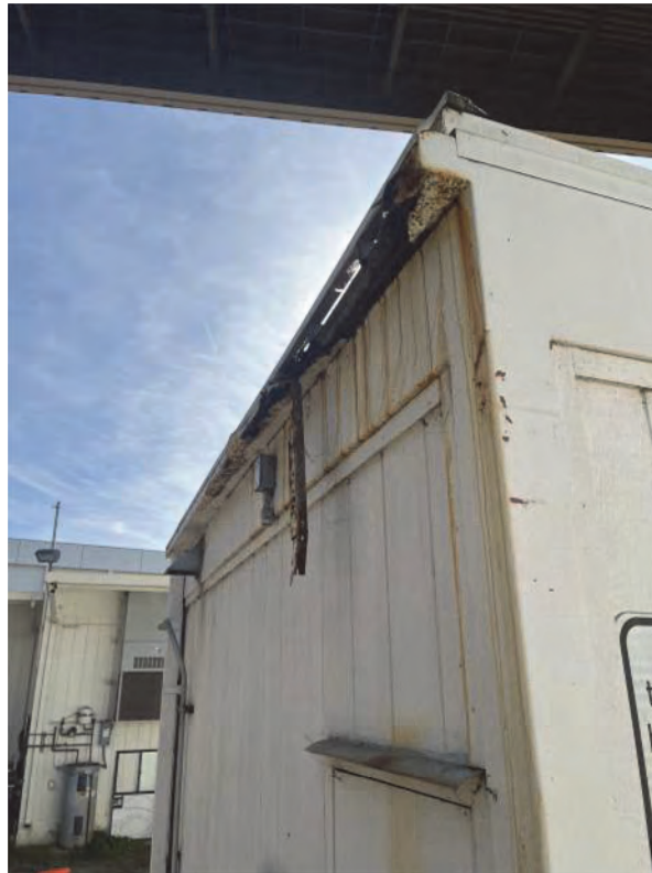
Significant Damage to Gutter
