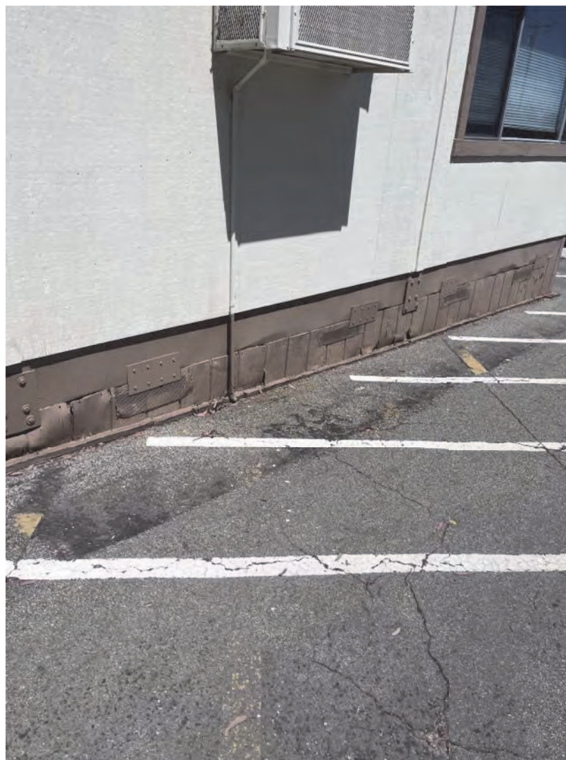
Slight Deterioration of Cripple Wall Sheathing
