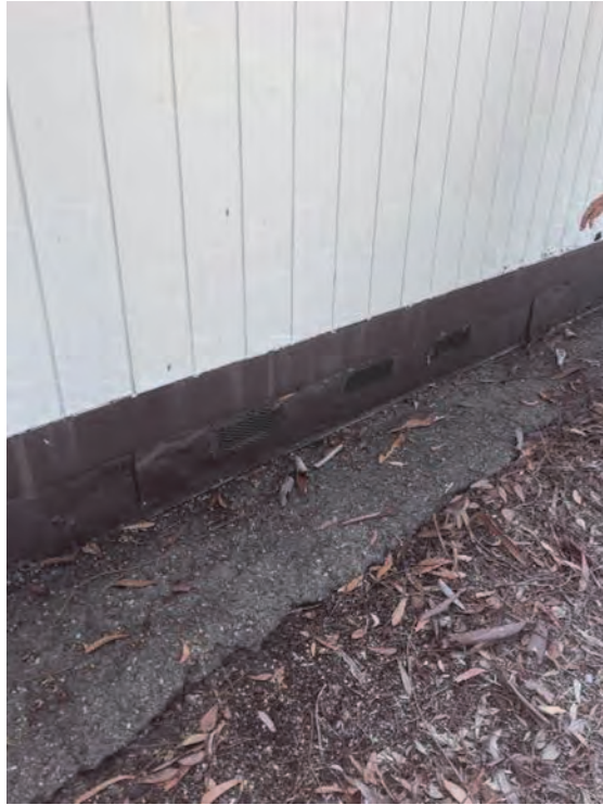
Slight Deterioration Cripple Wall Sheathing
