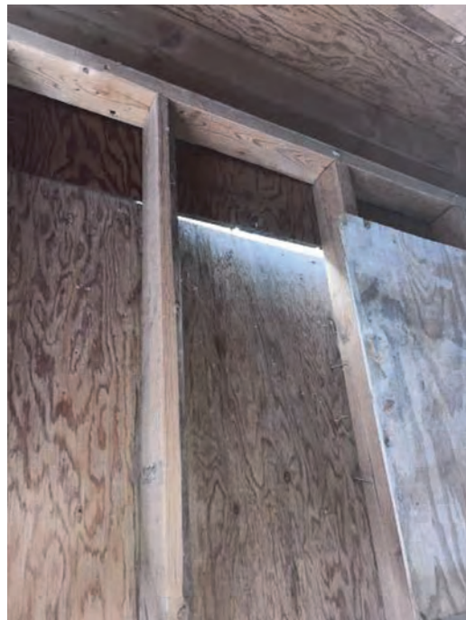
Building 37 - Damage to Exterior Wall Sheathing
