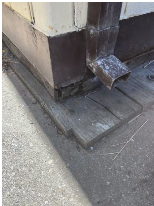
Damage to Plywood Skirting
