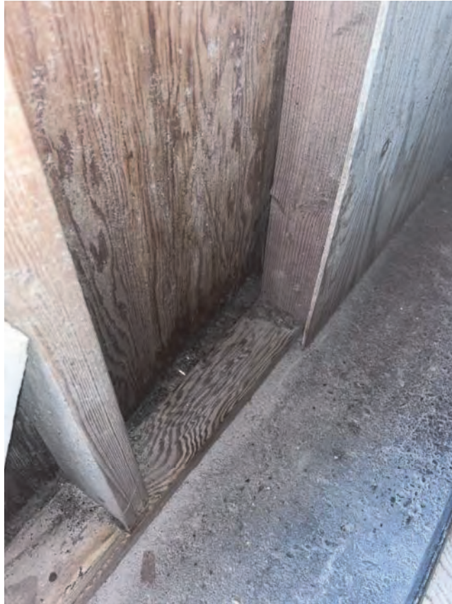
Building 37 - Damage to Sill Plate
