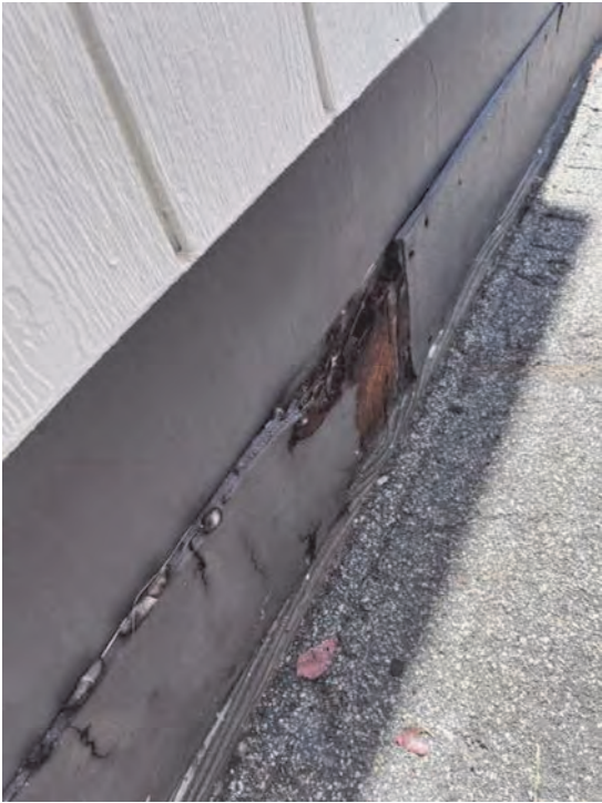
Damage to Plywood Skirting
