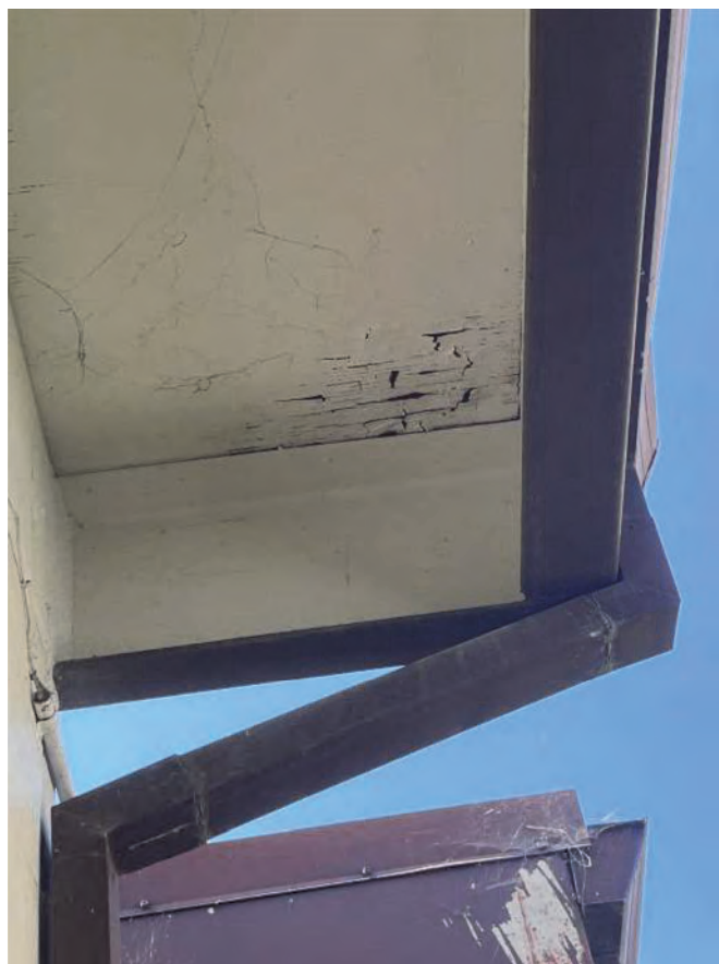
Damage to Plywood Roof Sheathing
