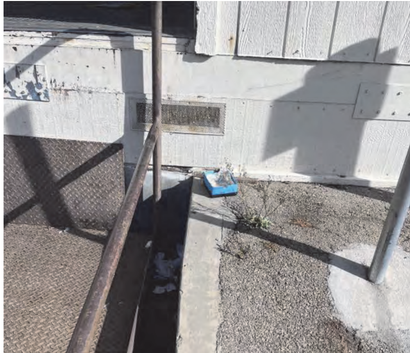
Deterioration of Wood Sill-On-Ground
