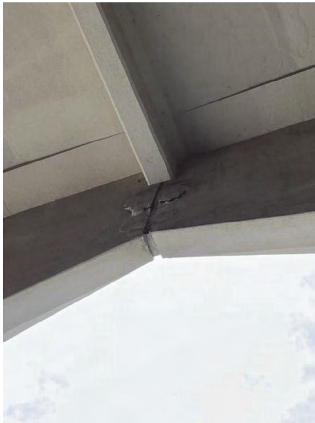
Water Damage at Connection of Precast Concrete Exterior Columns
