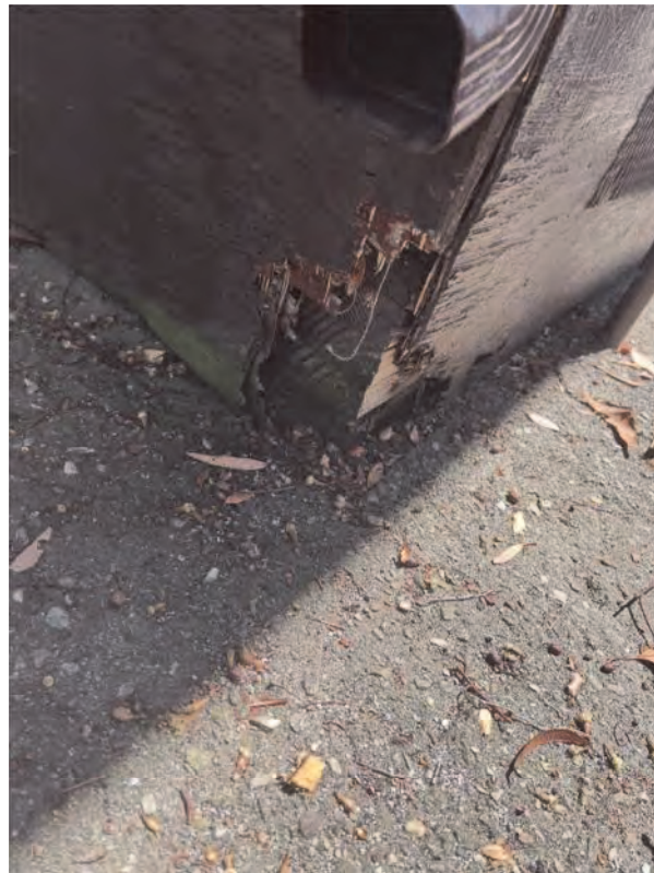
Slight Deterioration Cripple Wall Sheathing
