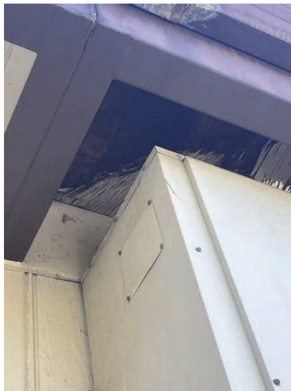
Damage to Plywood Roof Sheathing
