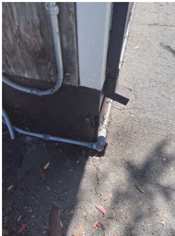
Slight Deterioration to Cripple Wall Sheathing
