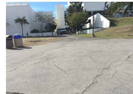
asphalt block cracking
