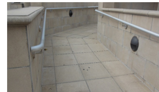
Ramp to building entry; intermediate landing exceeds 2% allowed maximum cross slope
