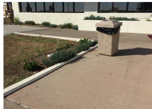
construction joint with sealant between concrete with exposed aggregate and concrete with integral color
