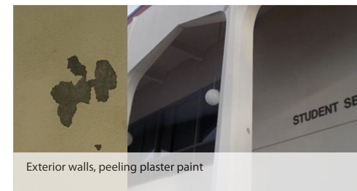
Damaged plaster and paint at corner
