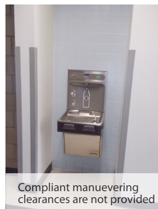
Accessible clear floor space not provided. Mirror and soap dispenser mounted above ADA compliant heights.
