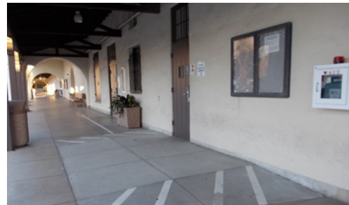
Path of travel interrupted by ramp
