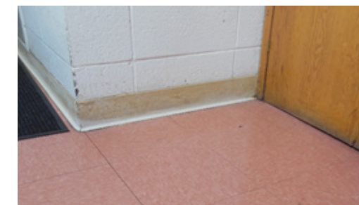
VCT in classrooms; worn and in need of replacement
