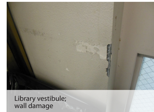
Library; lower level window sill vandalism and damage
