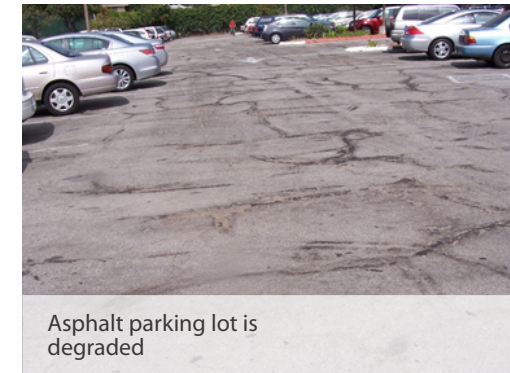
Accessible parking stalls are not compliant and striping is degraded
