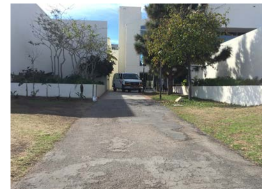
asphalt cracking and surface deterioration
