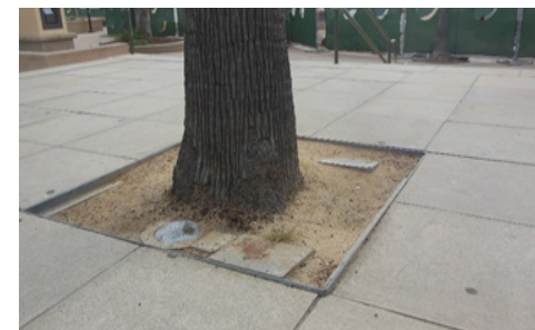
West entry plaza tree well; hazardous surface feature along path of travel.
