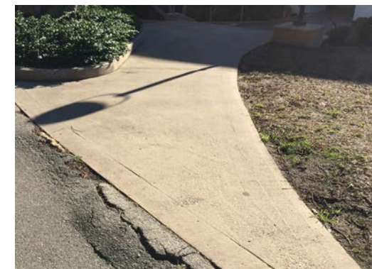
uneven surface and cracking at paving transition from asphalt to concrete
