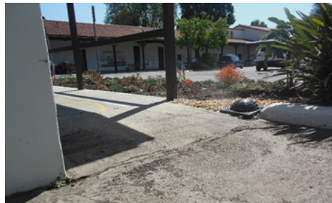
Path of travel with hazardous surface feature and no level landing at bottom of ramp
